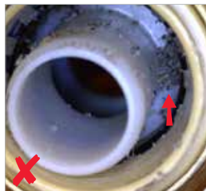
Dirt/debris inside fitting
