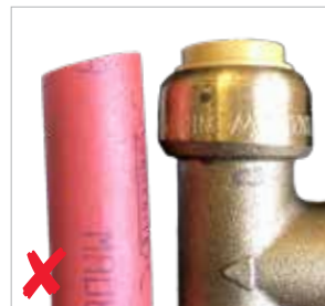
Pipe has not been cut square
